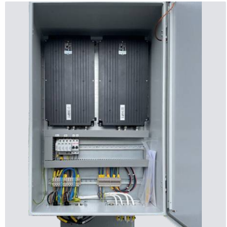
Control Gear put in the electric cabinet
