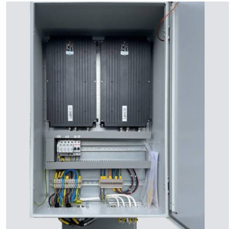
Control Gear put in the electric cabinet
